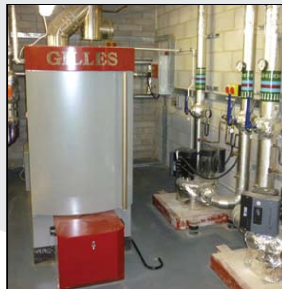
Woodchip pellet boiler with storage and automatic fuel transport system
