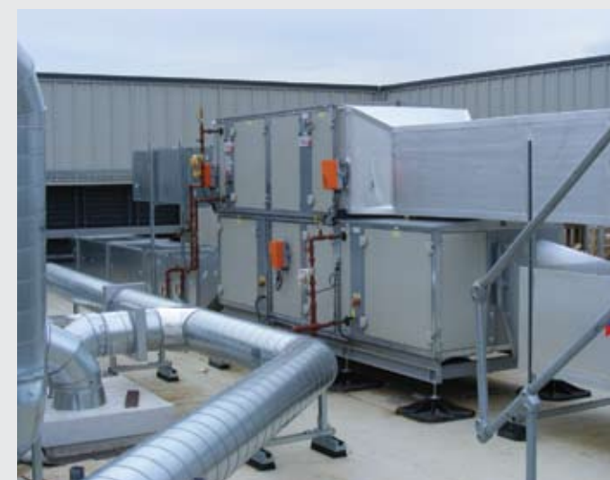
Roof mounted air handling plant at a city centre shopping arcade.
