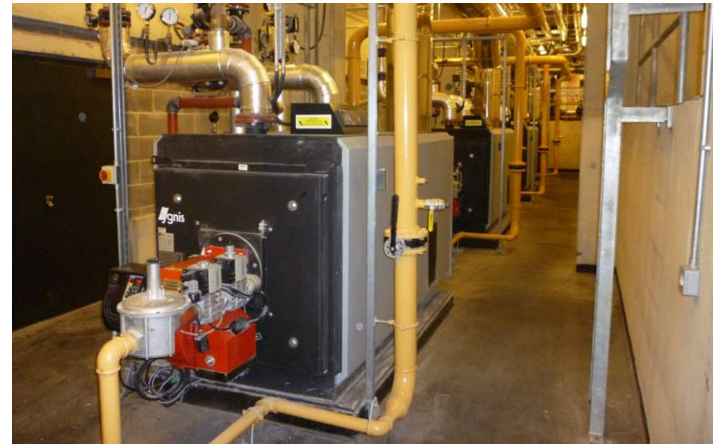
Gas fired boiler plant serving 326 apartments at One Park West
